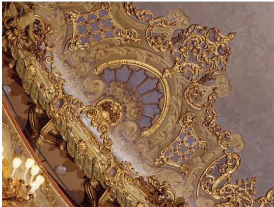
Detail of the ceiling in the Teatro La Fenice, Venice, before the fire of 1996
